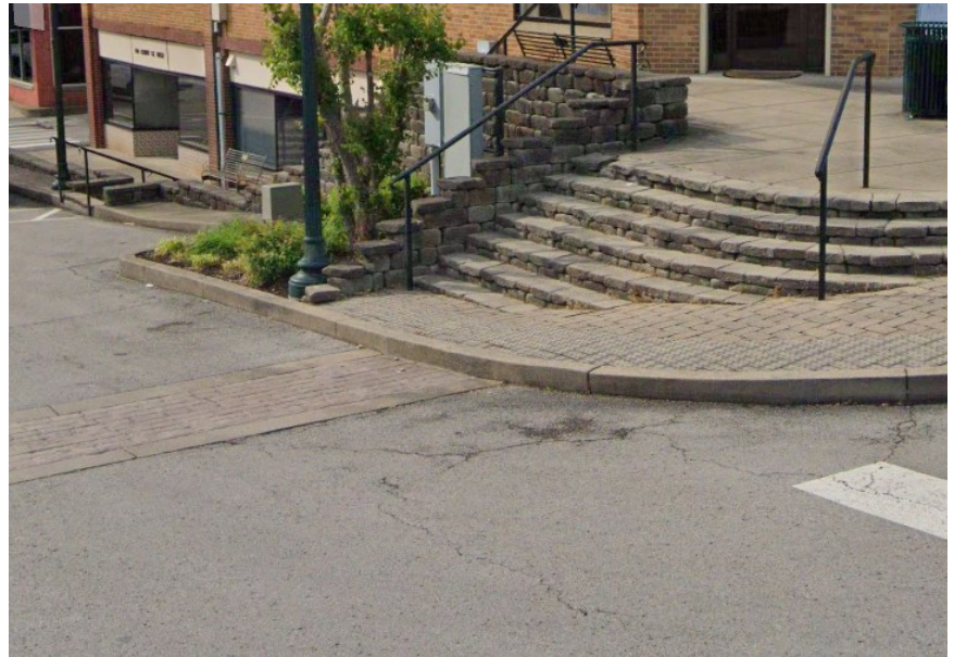
Example of ADA non-compliant intersection crossing at the intersection of Court Street and Main Street (US 68) in Greensburg, lacking correct ramp and detectable warnings. Photo courtesy of Google.
